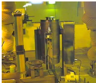
Vitrified Waste Canister Counter
